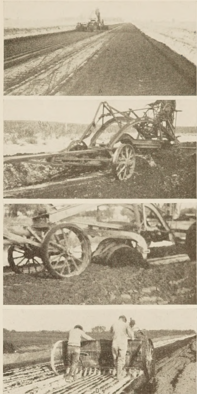
FIGURE 2.—APPEARANCE OF THE SURFACE DURING CONSTRUCTION. A, BLADE GRADER SPREADING THE TOP 2 INCHES OF THE SURFACE; THE REMAINING WINDROWS CONTAIN MATERIAL FOR THE SHOULDERS. B, THE EQUIPMENT USED WAS ILL-SUITED TO PERFORM THE WORK REQUIRED OF IT. C, IN COLD OR COOL WEATHER THE MIXTURE WAS TOO ROPY TO MIX WELL AND WAS PICKED UP BY THE WHEELS. D, SPREADING LIMESTONE DUST WITH A DRILL-TYPE SPREADER.
